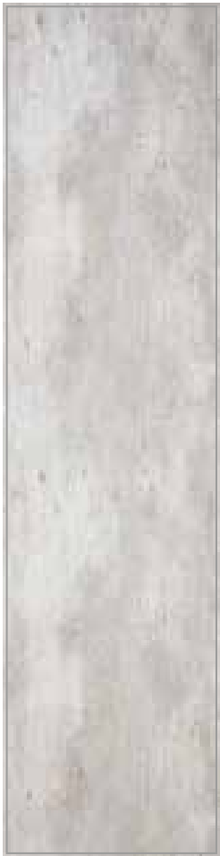
2204 S Cracked Cement
